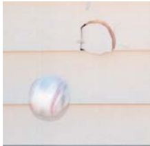
Unsupported vinyl siding
